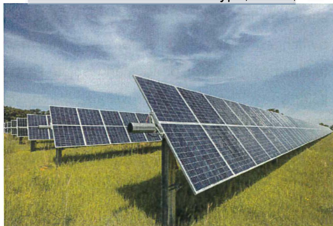
Figure 2. Mounted PV Modules
