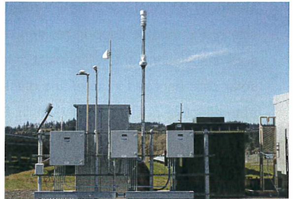
Figure 4. On-site electrical infrastructure
